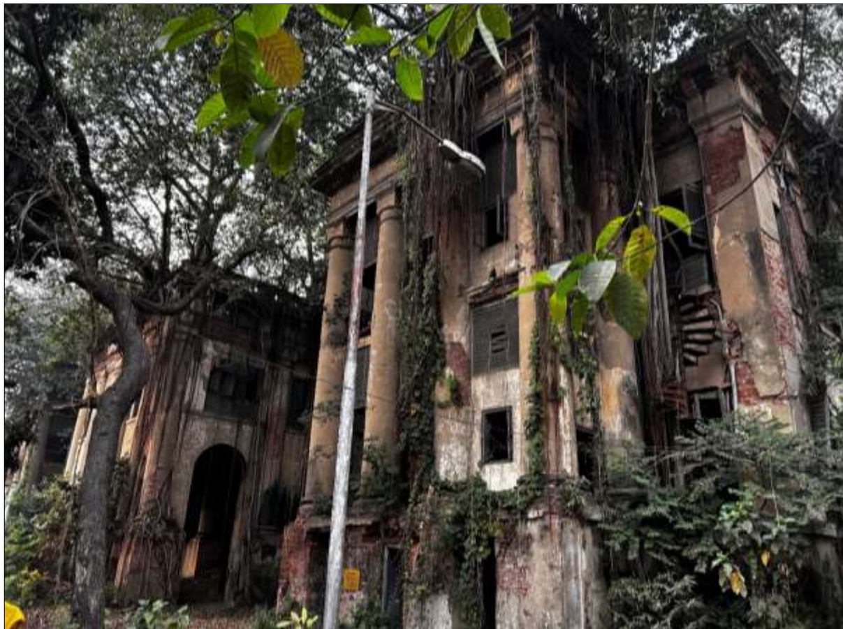
Figure 23: The state of the old Free Church Institution building at 74 Nimtala Ghat Street, Kolkata, on 18 February 2025 (photograph: R.C. Kapoor).
