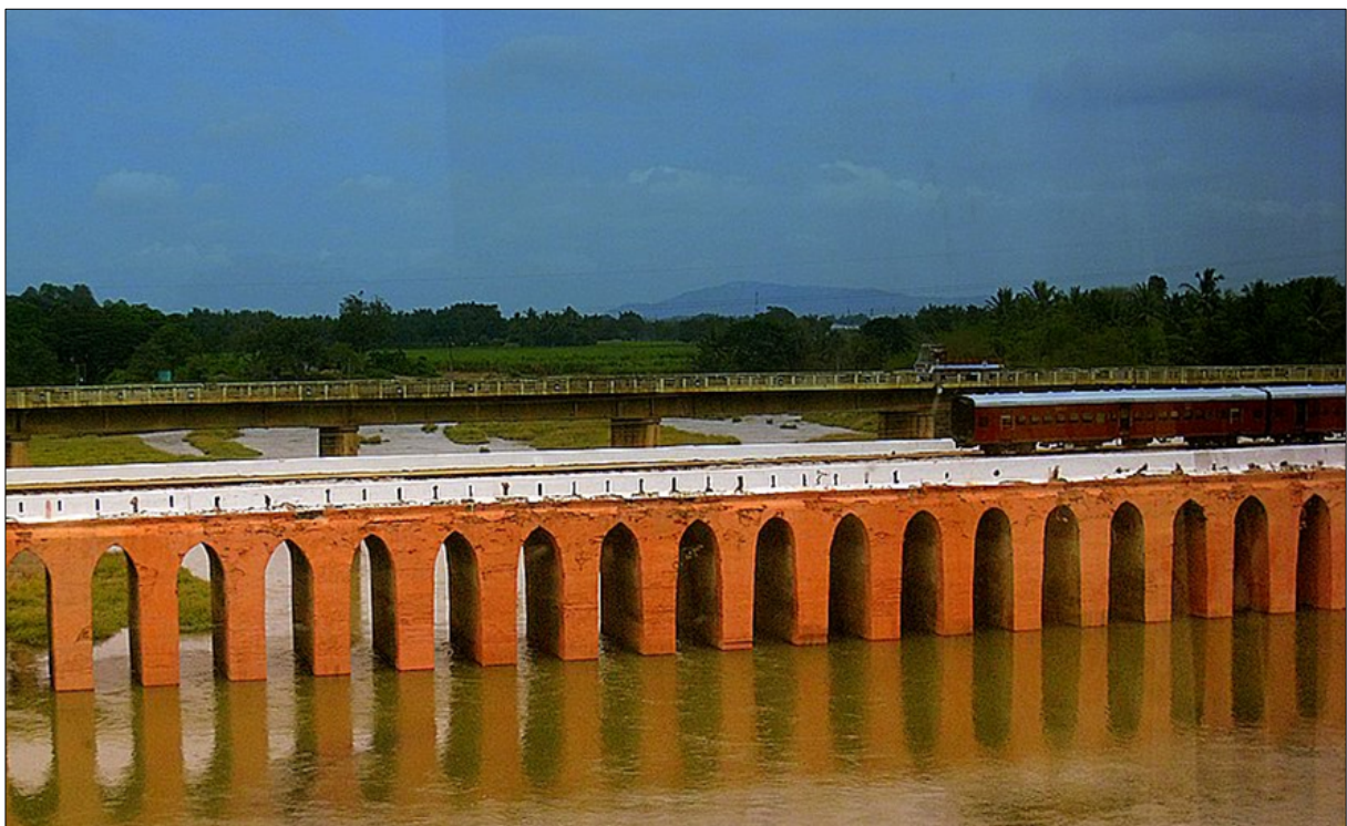
Figure 13: The Kabini Bridge, Nanjangud (2011 image by Suraj, TS; adapted from Wikimedia Commons).
