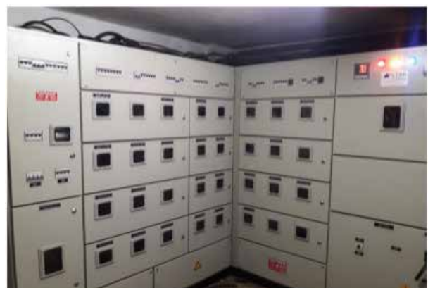
Figure 4.1: The installation of new LT metering panel at the staff quarters at Banasawadi road, Bengaluru.
