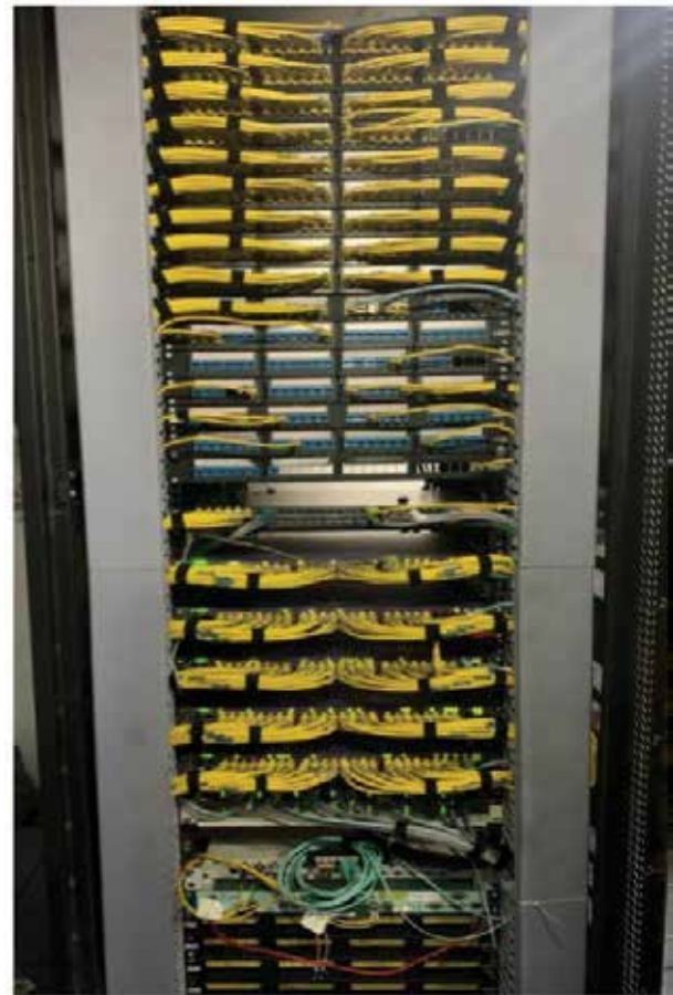
Figure 4.9: Network Rack at IIA Computer center.
