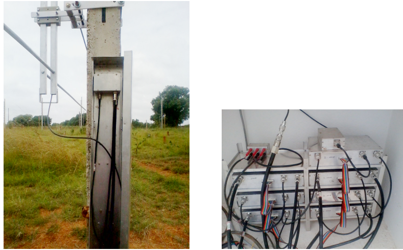
Figure 2.15: The left photograph shows the pre-amplifier connection. It is kept in a rectangular casing to protect from pests. The right photograph shows the RF modules (the group amplifier, filters, DSB boxes, their control signal units and the AC mains power supply) inside the RCC box. Individual signals from the antennas are brought to the RCC box through low-loss coaxial cables before being added using DSB modules at various stages (I, II and III).
