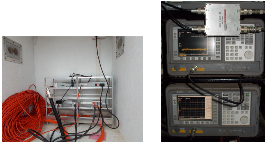
Figure 5.3: The left inset picture shows the RCC protective casing for RF & RF to Optical conversion modules. Here the main/second stage amplifier is also protected by lightning arrester (not in picture). The rolled orange cable is the optical fibre ( \approx 500 m) which transport the modulated wideband RF from the converter to lab. Similar optical to RF modules at lab side demodulates the optical to wideband RF and later connected to the 4-port phase quadrature and finally to two independent spectrum analyzers that are connected to independent PCs via PCI-GPIB interface (refer Section 2.6.3).
