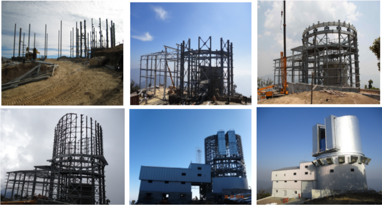
Figure 4: Snapshots of telescope enclosure building at Devasthal are shown since the beginning of construction in September 2012 till its completion for telescope installation in June 2014, respectively left to right.
