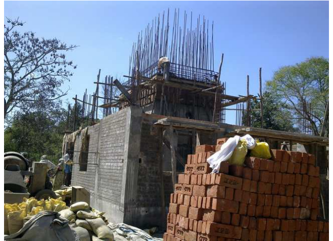
Figure 2.11: Pier upto a height of about 4.5 metres surrounded by the outer structure upto ground floor (February 2011).
