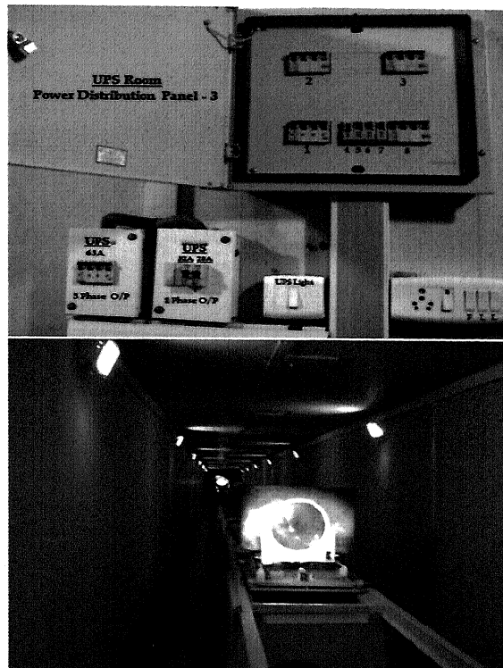
Modified solar power control panels and interior view of renovated Solar Tunnel Telescope.
