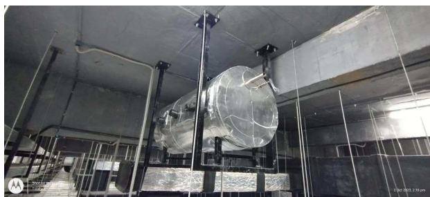
Figure 4.20: 250 lt capacity hot water generator at ITOFF.
