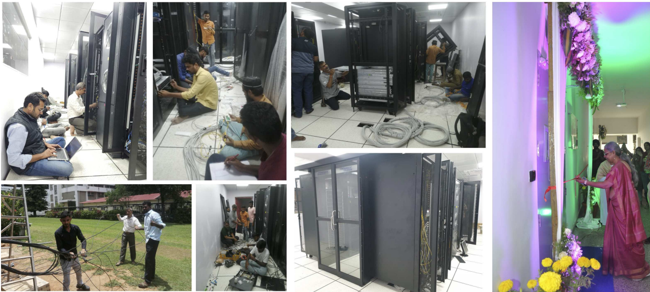
Figure 6.11: Migration of IT infrastructure and services to the new Data Center.
