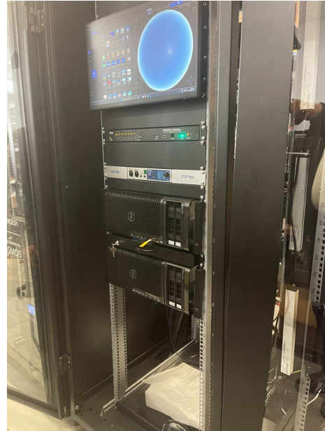
Figure 5.13: Prototype of server rack at RSA Cosmos, France.
