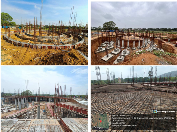
Figure 5.10: Clockwise from top left: Ring beams; ring beam columns footing level; re-inforcement for ground floor slabcasting; and columns raised upto ground floor slab level.
