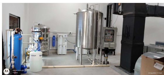
Figure 4.17: De-ionised water plant at CREST.
