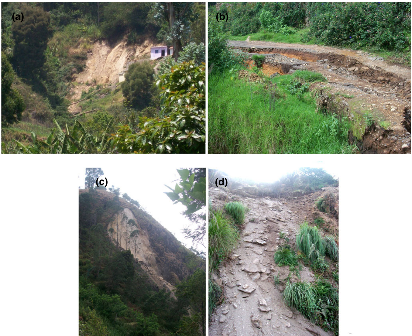
Figure 3. Examples of Landslide in Study area at (a) Munjikal, (b) & (c) Kodaikkanal town and (d) Kovilpatti.
