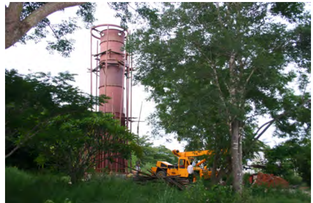
Figure 2.11: Erection of the DIMM tower at VBO. The separate steel cylinder (pier) and outer pipe structure are seen.
